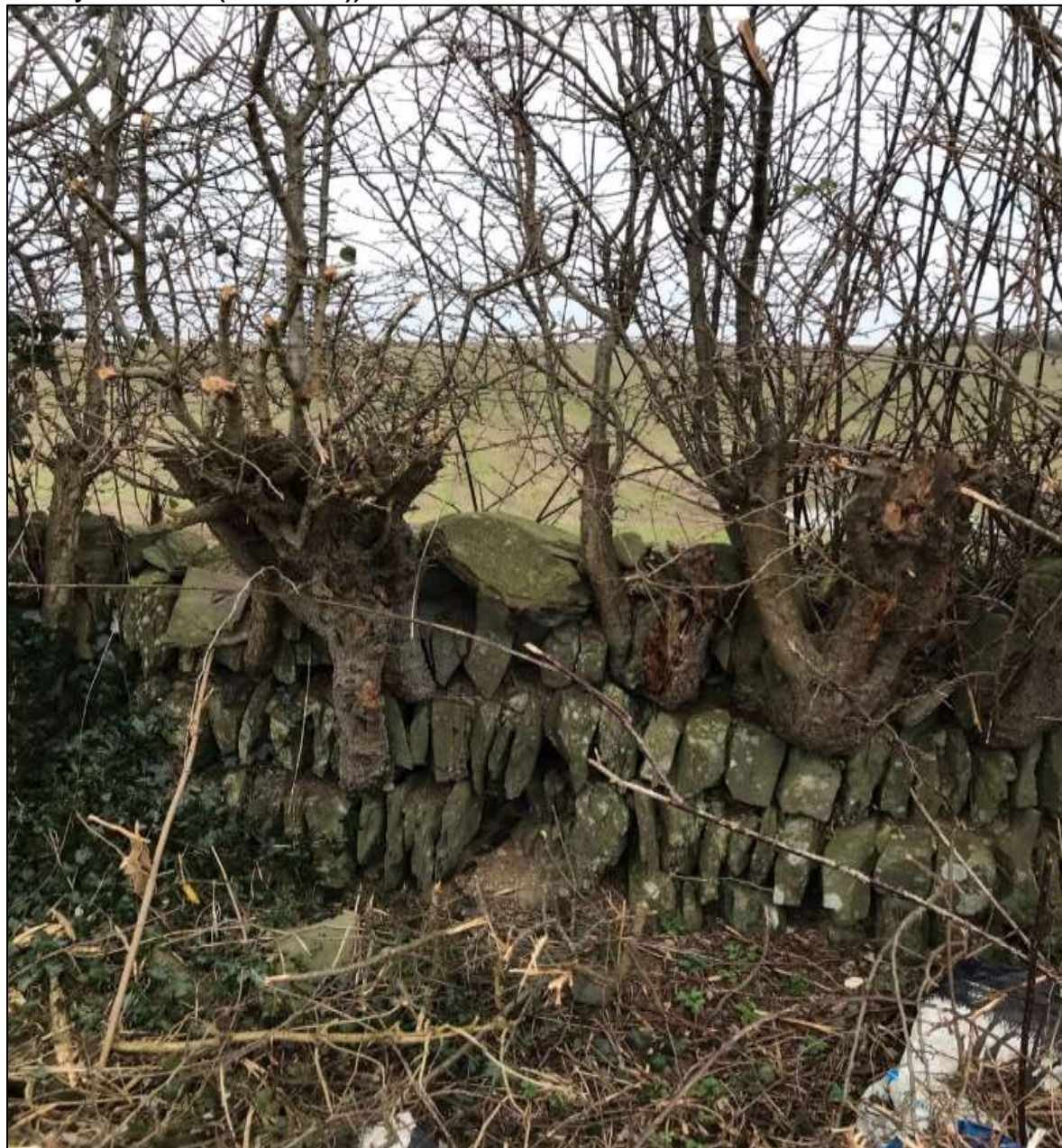
Plate 10-3: The hedgerows are characterised by old stone walls with coppiced hedges (in vicinity of the Site (PR21 / 631)).
